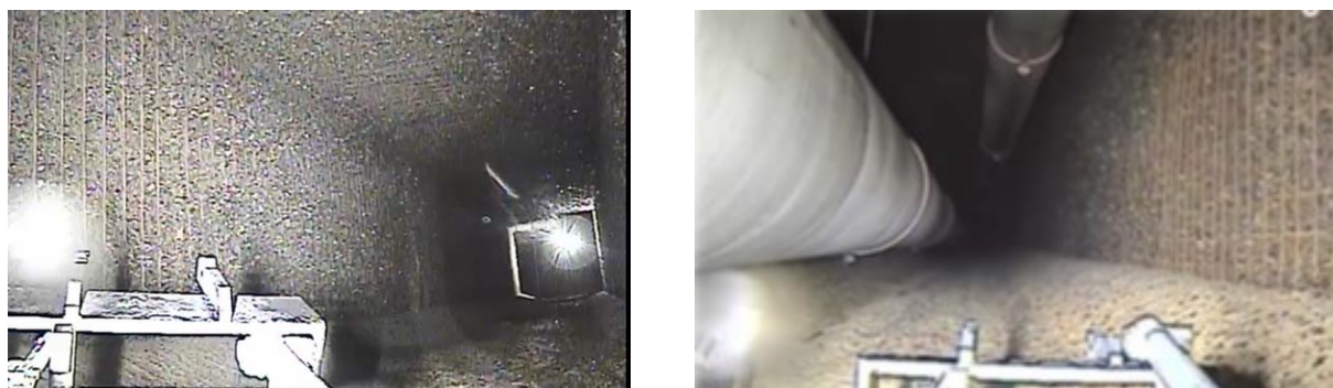
Fig. 5 – Recent tunnel inspections showing concrete erosion and exposed rebar
