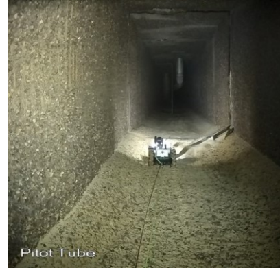
Fig. 18 - Pitot Tube Port Camera View
