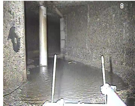
Fig. 2 - Standing water in CAEX Tunnel
