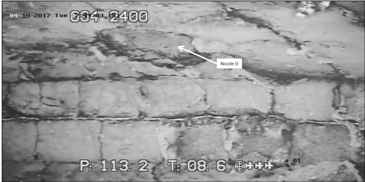
Figure 5-6. Vapor space refractory condition
