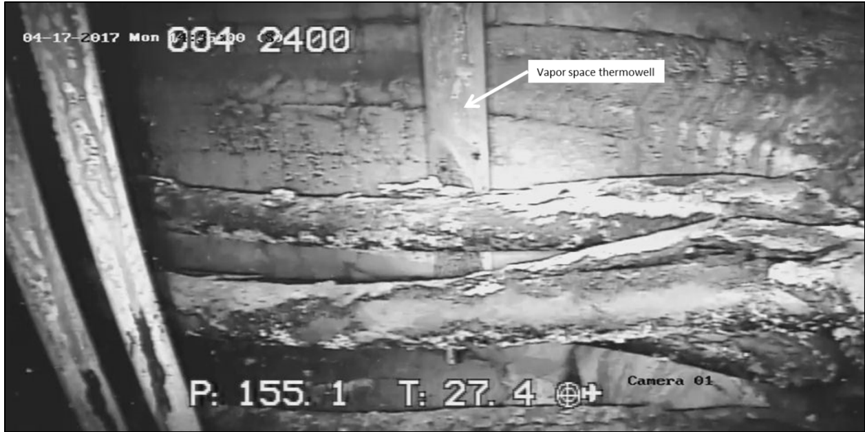
Figure 5-18. Deformation of dome heaters, east side of melter
