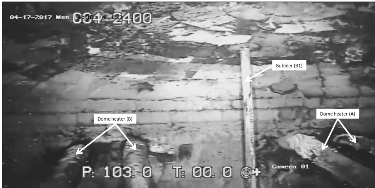
Figure 5-2. Melter 2 vapor space refractory and dome heaters
