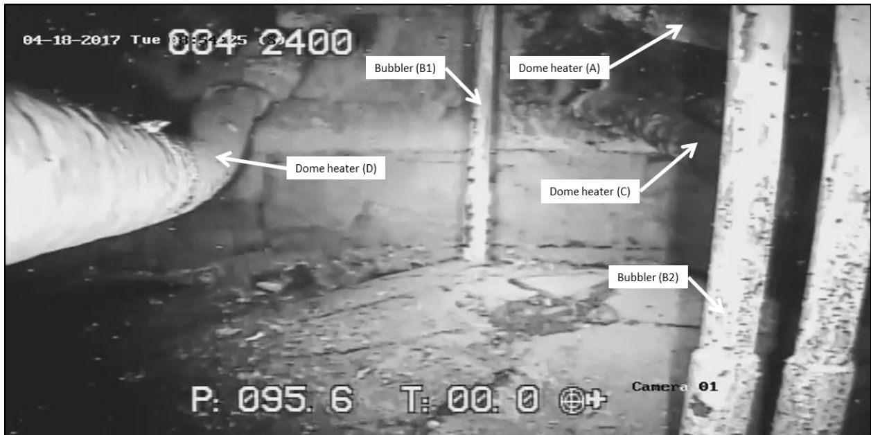
Figure 5-21. View along dome heaters showing deformation, lower pair, west side of melter
