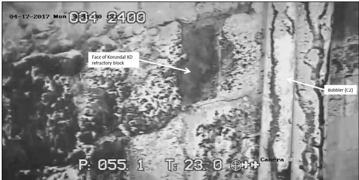
Figure 5-4. Exposed face of Korundal XD vapor space refractory near Bubbler C2
