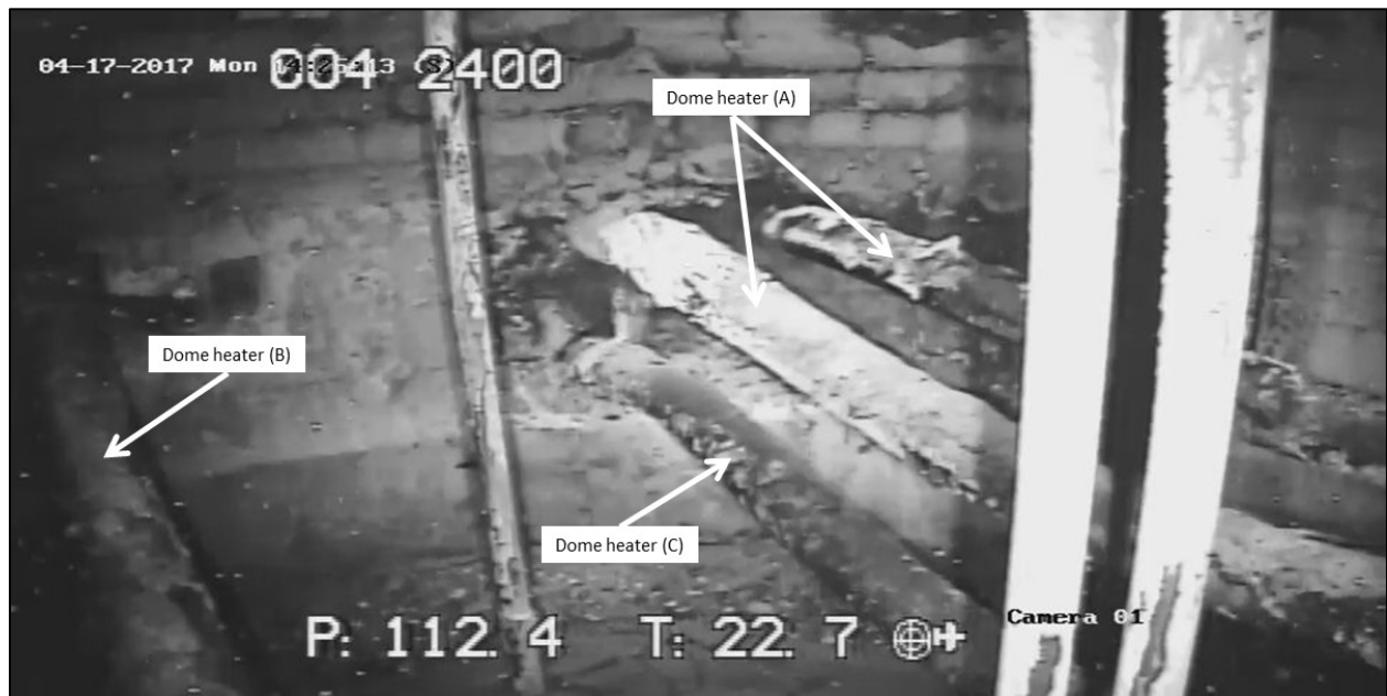
Figure 5-10. Dome heater penetrations, northeast side of melter
