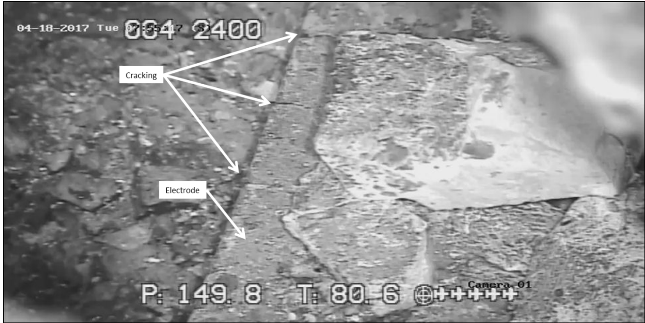
Figure 5-27. Detail view of cracks visible on top of upper electrode, southeast side of melter
