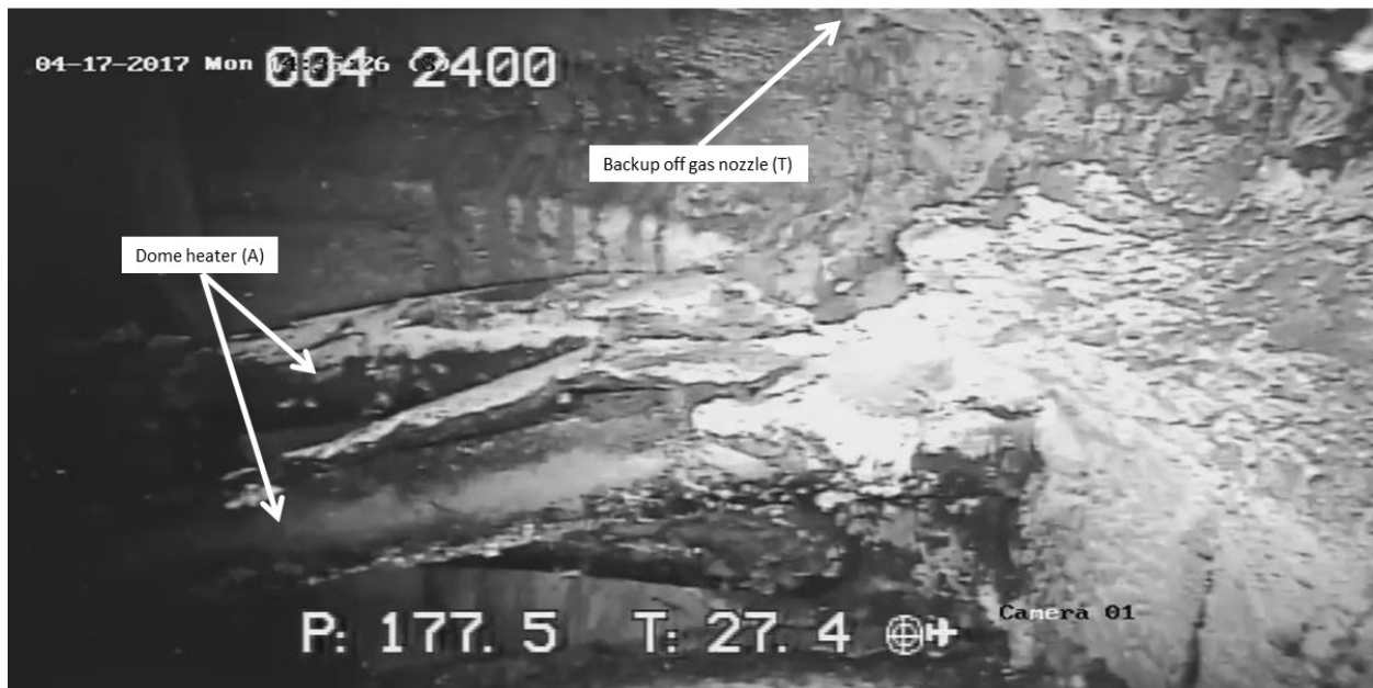
Figure 5-14. Dome heater penetrations, upper pair, southeast side of melter
