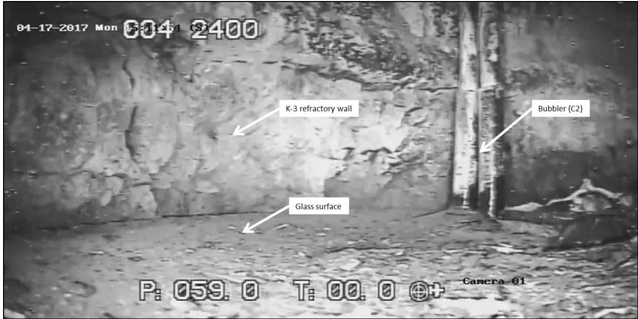
Figure 5-33. Glass contact refractory at melt line, west side of melter
