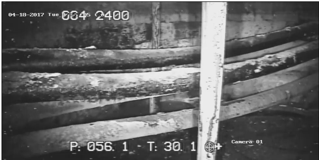
Figure 5-19. Deformation of dome heaters, west side of melter
