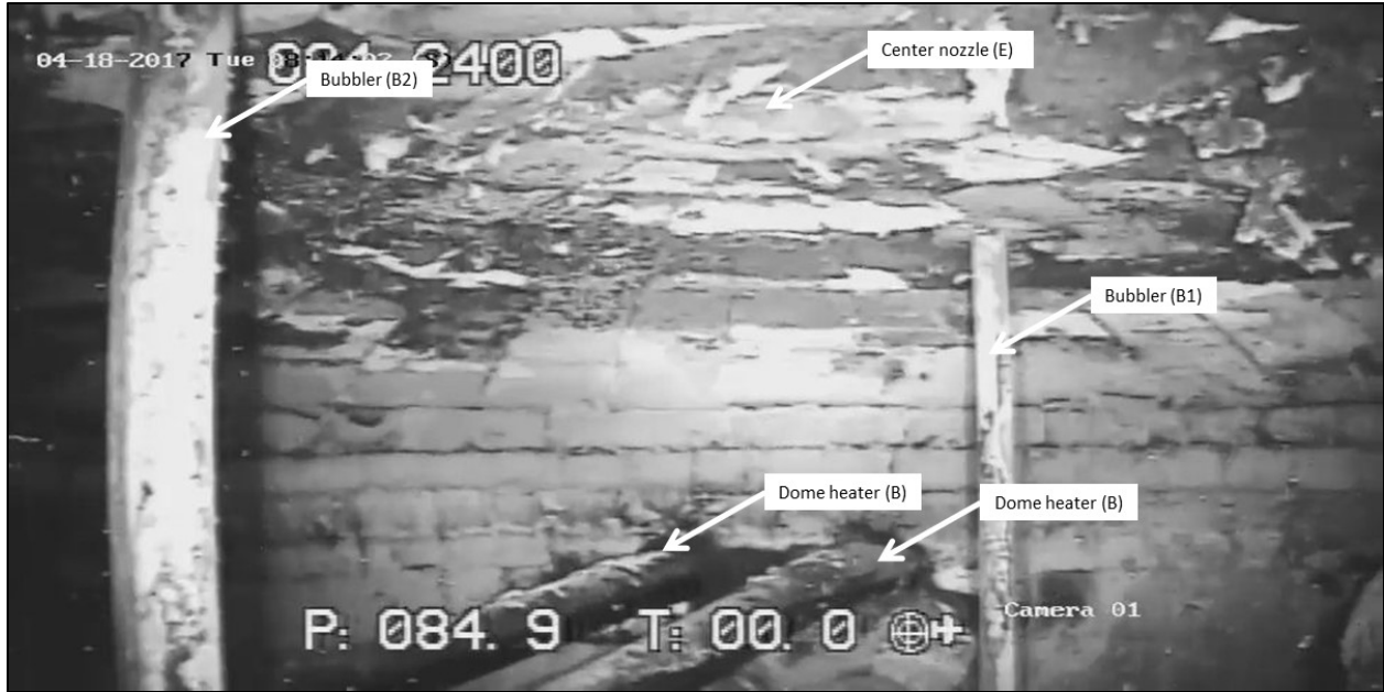
Figure 5-1. Overview of Melter 2 vapor space refractory and components
