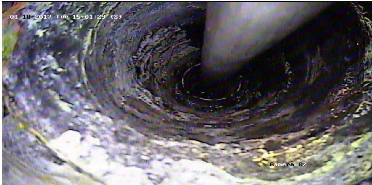
Figure 7-2. Closer view of pour spout showing region of removable insert with inspection camera system inserted
