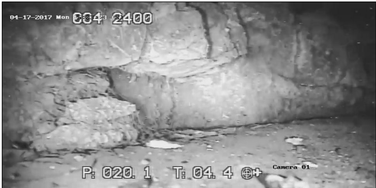
Figure 5-34. Second view of glass contact refractory at melt line, west side of melter
