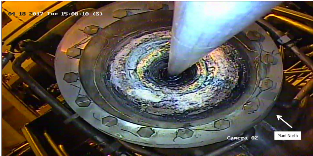
Figure 7-1. View of pour spout looking up toward top of melt cell with inspection camera system inserted
