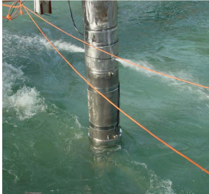
Figure 3. Submersible Mixer Pump during acceptance testing at the SRS Full Tank Facility.
