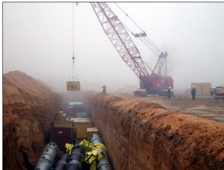
Figure 6. E-Area Slit Trench Facility showing a range of waste materials. Also note the red clayey sediment, characteristic of the upper sediment strata.
