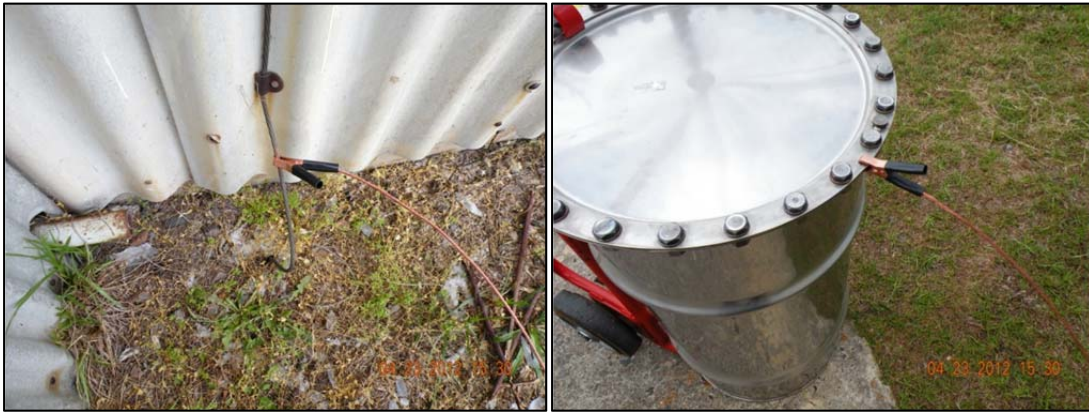
Figure 6-7. Grounding wire connection (Left) and connection to Model 9975 package (Right).
