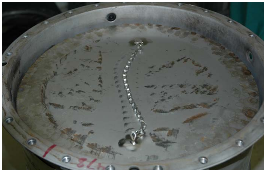
Figure 2. Water stains and other markings on air shield and upper drum interior. Photo taken by NMM personnel.
