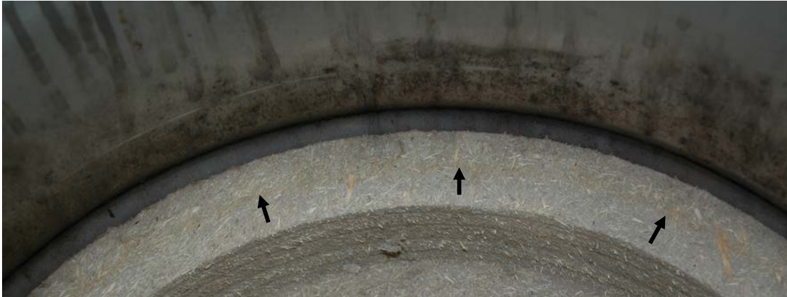
Figure 3. Water stains and other staining on drum interior. Light water staining is also visible on the step of the lower fiberboard assembly. Photo taken by NMM personnel.
