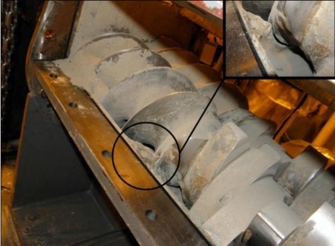
Figure 1-2. Grout build up at the auger/paddle interface in the saltstone 10-inch mixer 6
