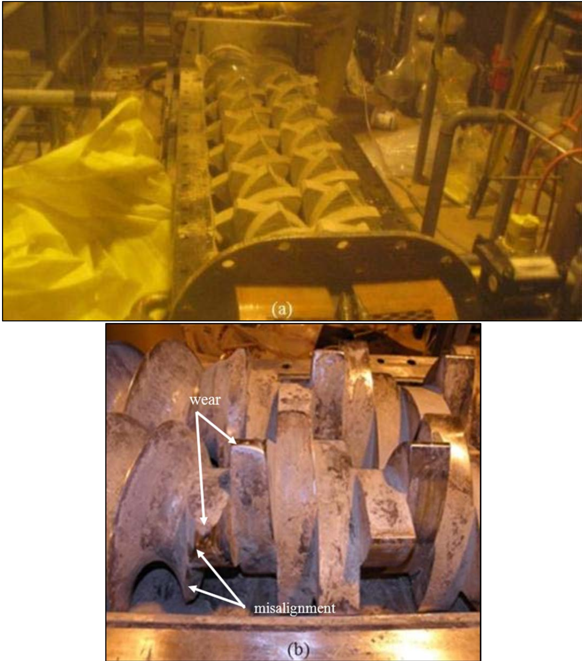
Figure 1-1. Inspection of the 10-inch Readco-Kurimoto mixer in the SPF showing (a) all the flat mixer paddles (note the tight clearance between the paddles and barrel), and (b) the misalignment of the auger and the first paddle as well as the wear on the last auger flights and first paddles 5,6
