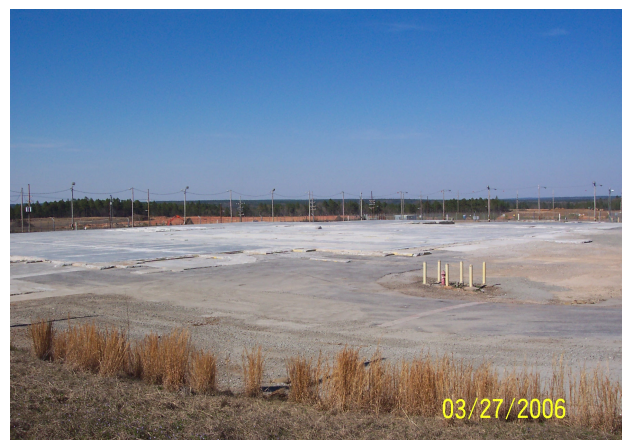
Fig. 3. Building 247-F after decommissioning, seen from perspective as in Fig. 2. Note location of yellow bollards in both figures.
